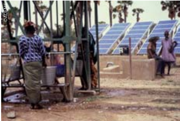
Solar for water pumping
