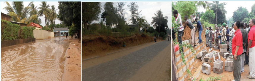
Water Erosion Infrastructure Destroyed Construction of Wall. Finished Water The Municipal Council and citizenry of Xai Xai have the tool and capacity to address soil erosion and its consequential damage to infrastructure and personal property as a climate change adaptation measure.
