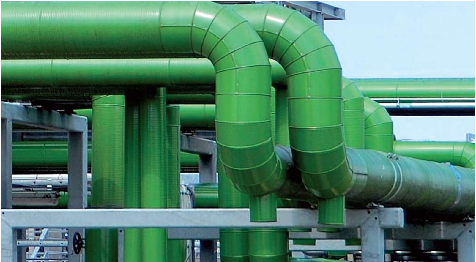
Steam pipes from a power plant and ethanol upgrading facility for reuse at the Kalundborg Symbiosis Industrial zone in Denmark.
