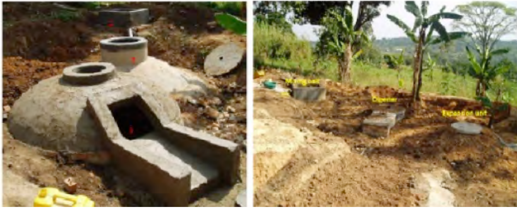
Figure 9: Fixed dome biogas digester in Buwambo
