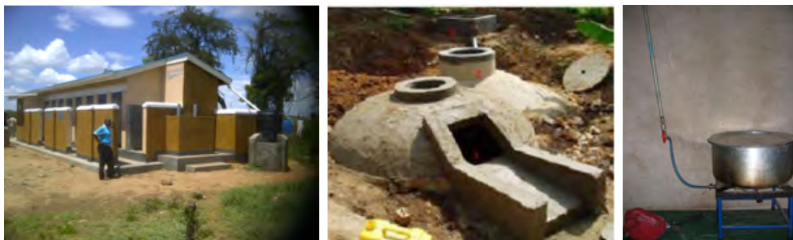
Figure 16: Composition of the bio-latrine technology: bio-latrine, biodigester, and gas cookstove
