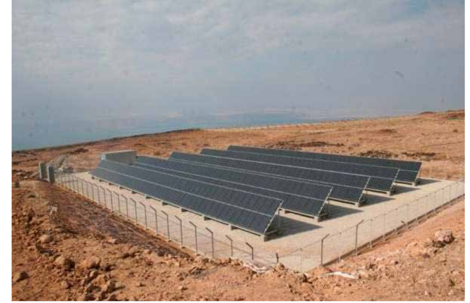
Figure 8. Grid connected to 100 kWp PV system at Dead Sea panoramic complex
