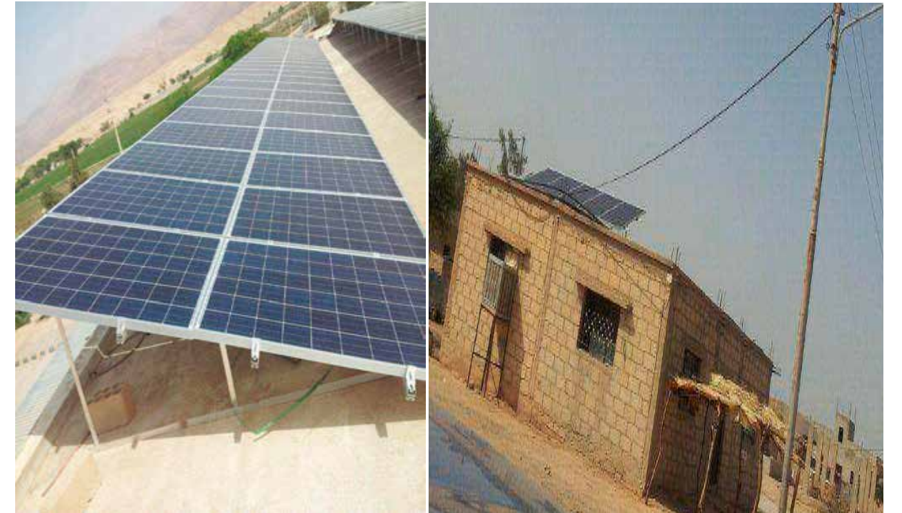
Figure 20. An example of installed PV system
