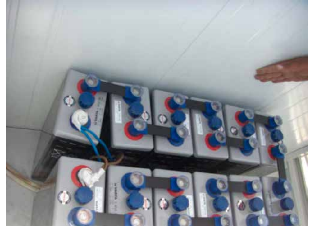
Figure 3. A new battery bank installed for each solar home system
