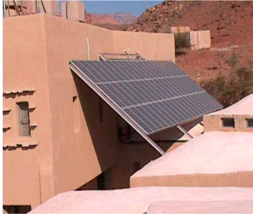
Figure 5. PV generator 4.5 kWp at the lodge
