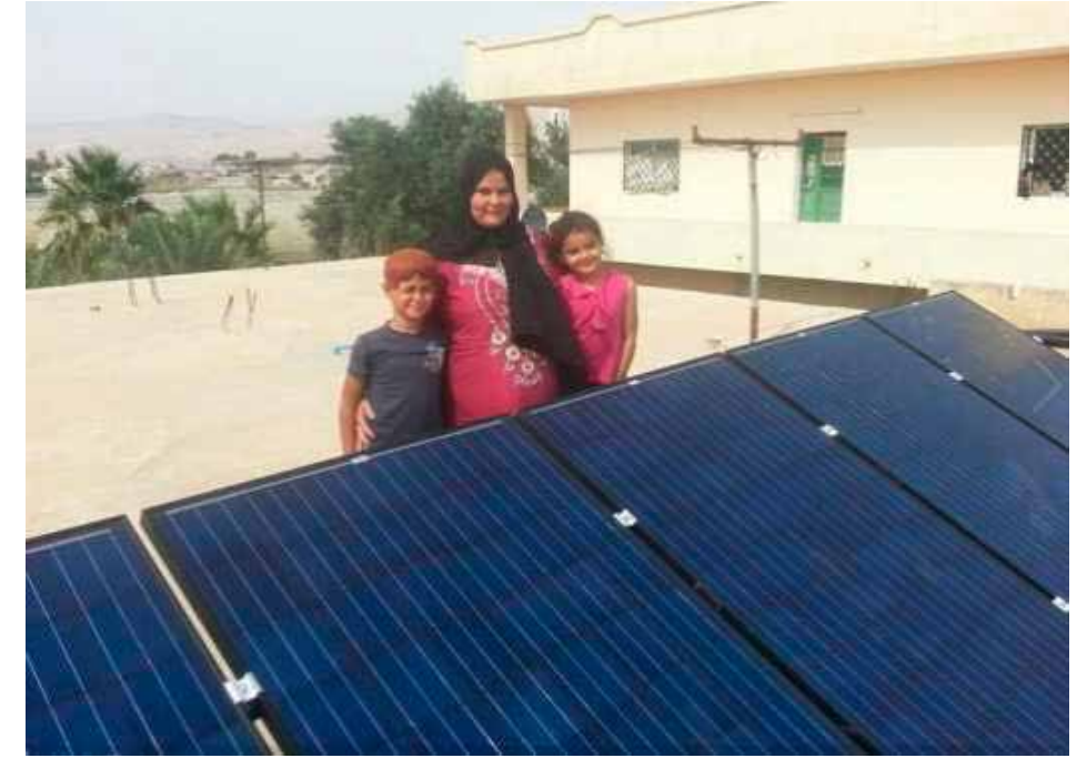
Figure 13. An example of a PV system
