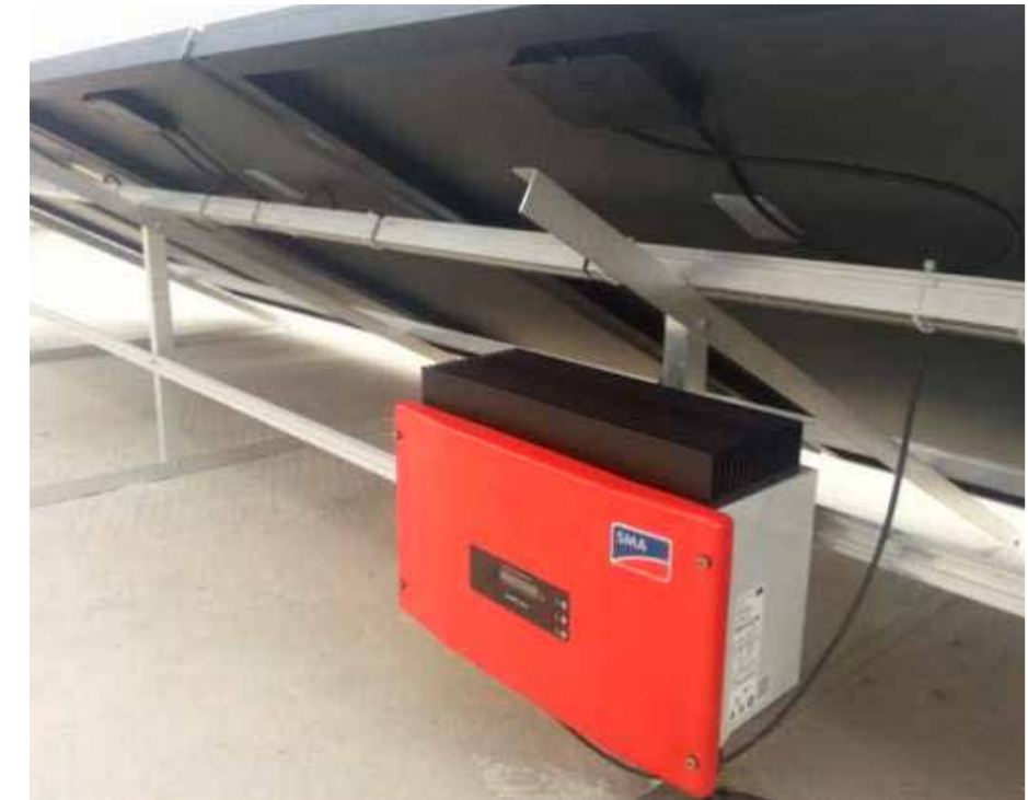
Figure 14. Grid-connected inverter installed outdoors
