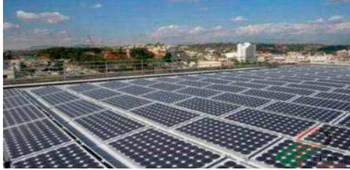
Figure 16. An installed PV system
