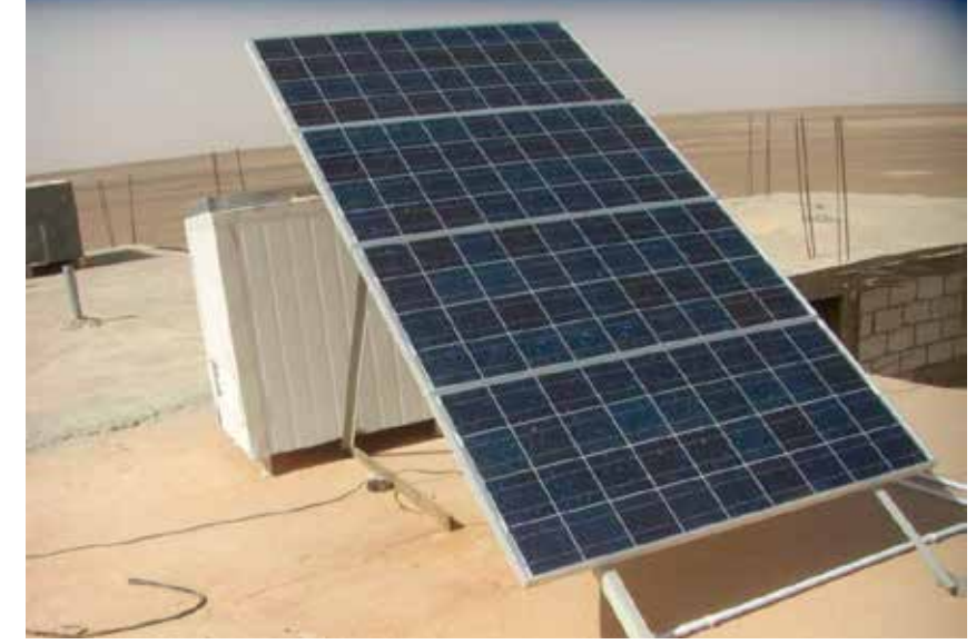
Figure 2. Solar home system 400Wp
