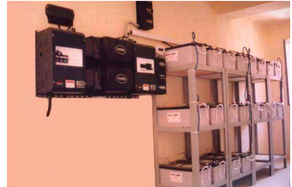
Figure 7. Battery banks and power conditioning units
